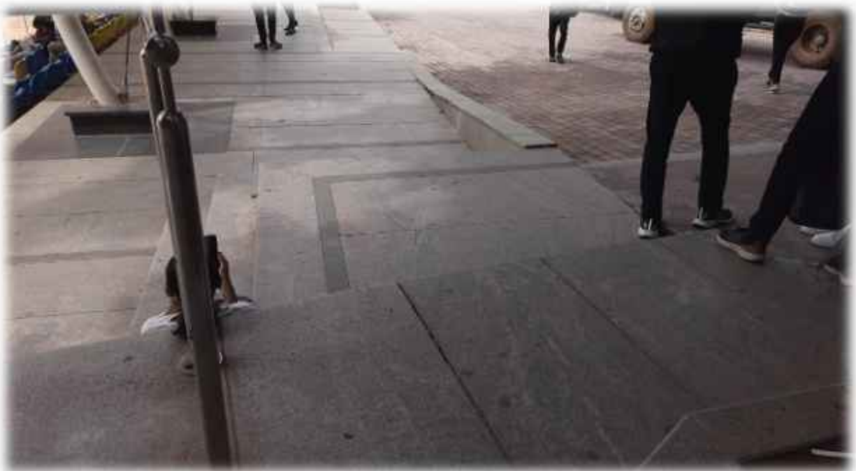
Ramp for differently abled students and others to enter in the campus
