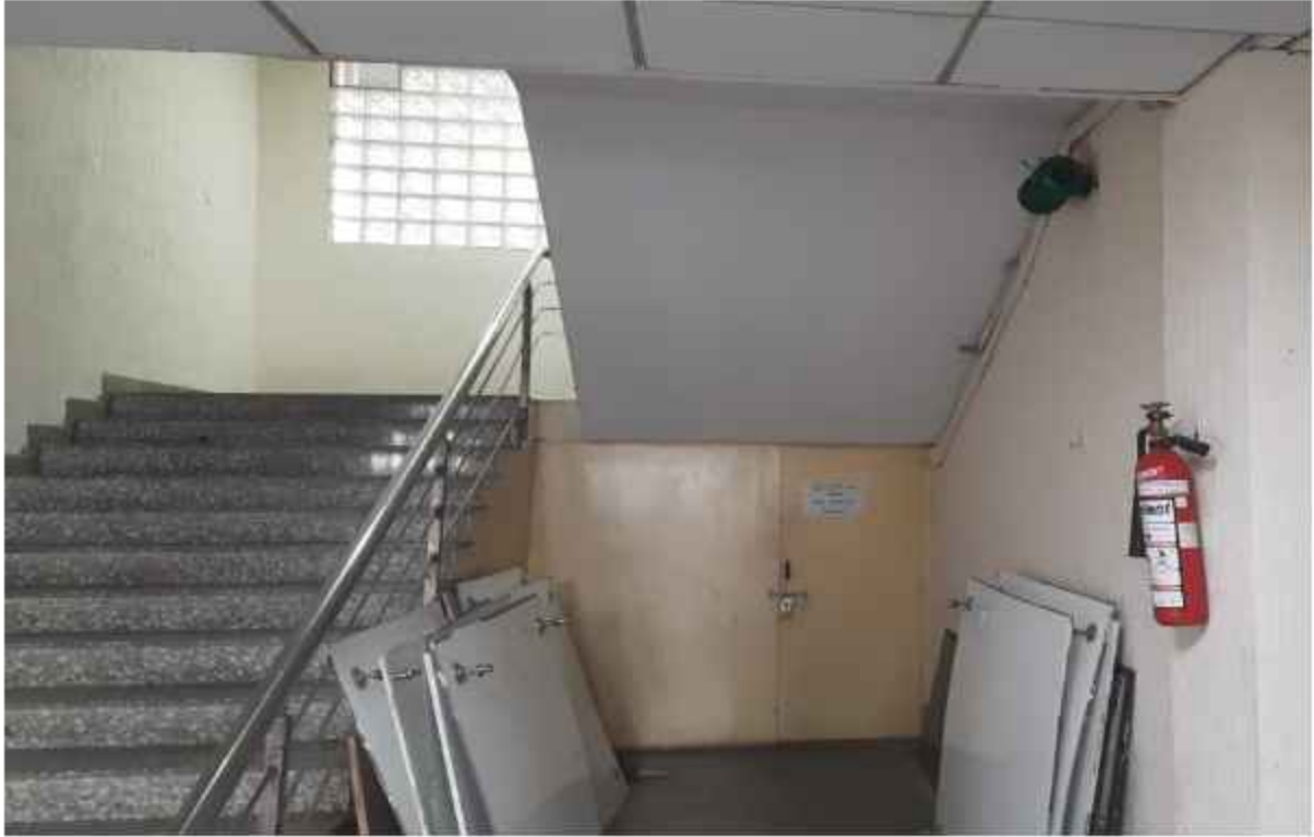
Fire Extinguisher along with Warning Buzzer/Alarm
