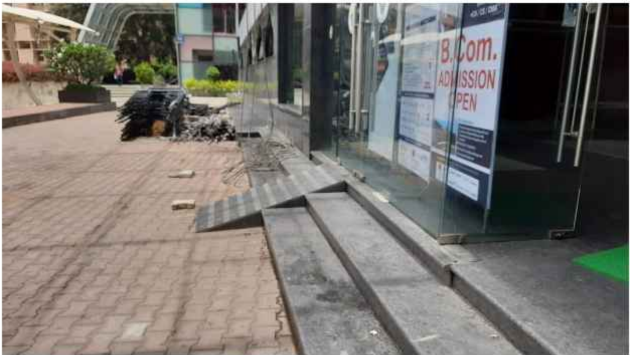
Ramp for differently abled students and others to enter in the building
